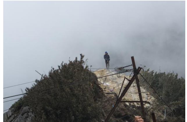
Drilling into the rocks with a jackhammer on the peak of mount Fansipan (March 2016)
