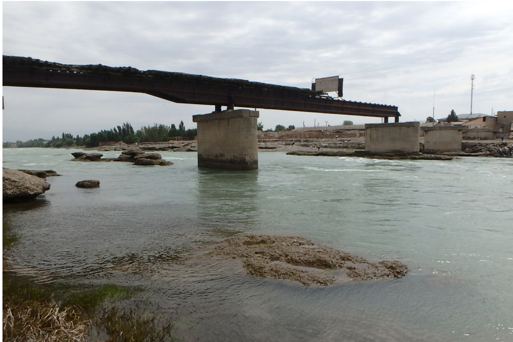
Bridge blown up between Kyrgyzstan and Uzbekistan. © Gulzat Baialieva
